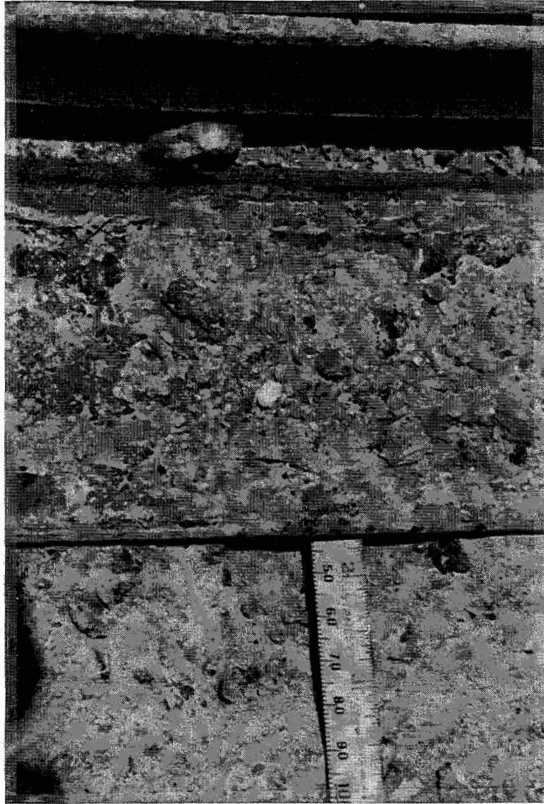
Figure 10 Depth of hole along top rail of joint
