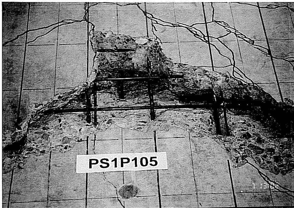
Figure 8.1: Bottom of precast prestressed panel Static Test Specimen #1 showing a portion of the punching shear failure plane and panel reinforcement.
