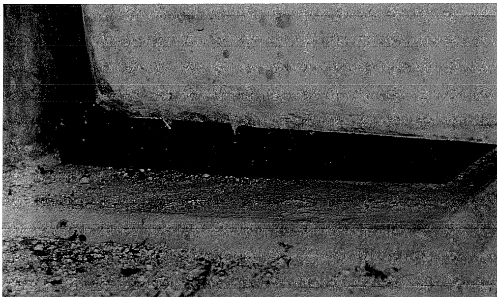
Figure 6- 1 Photo of bearing pad slip in Texas
