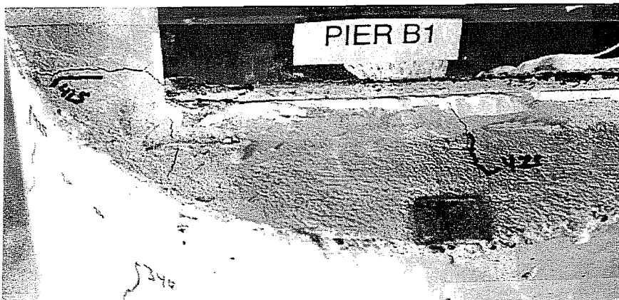
Figure 11-21 Splitting cracks due to bond distress in Specimen B
