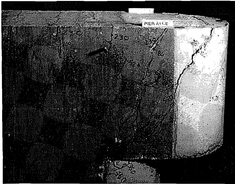
Figure 3.4 Crack Distribution on the Face of Pier A1-1 After Failure
