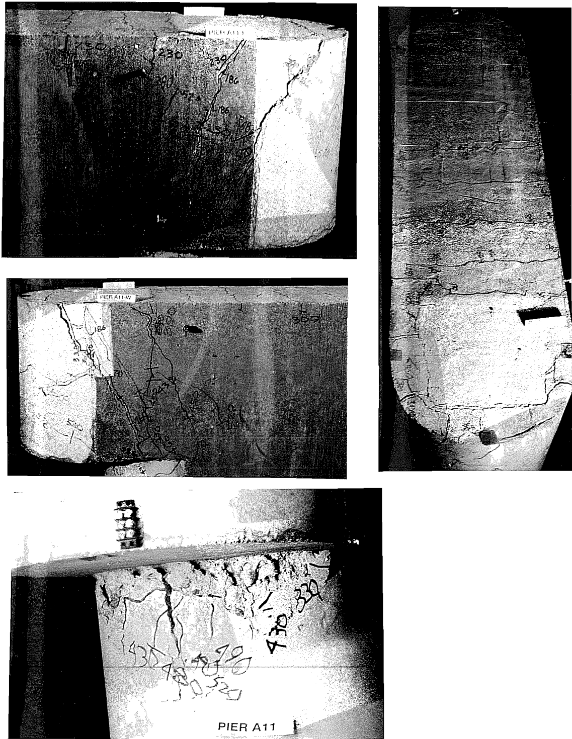
Figure C.1 Damage to Pier A1-1 After Failure
