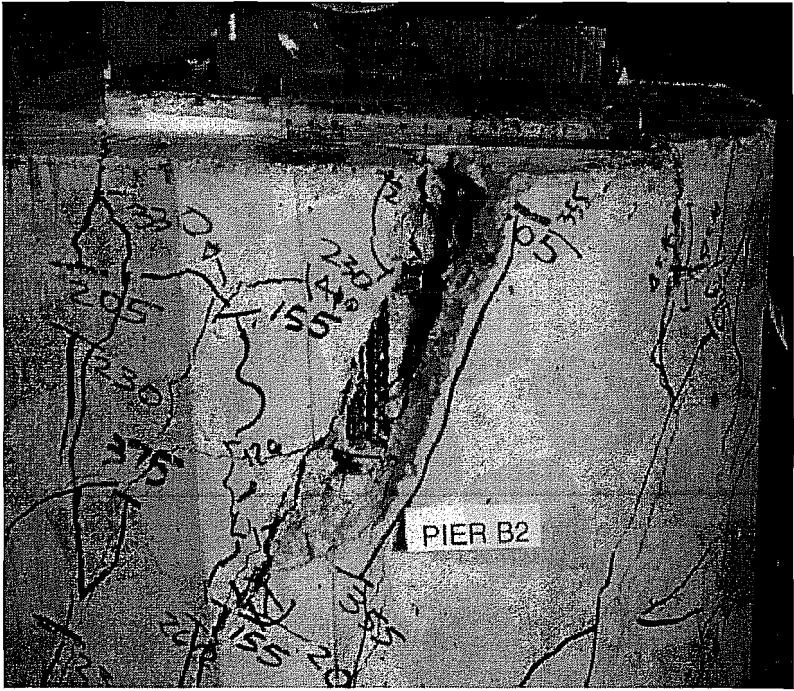
Figure 3.14 Opening of Flexure/Shear for Pier B-2 - Spalled Cover Removed
