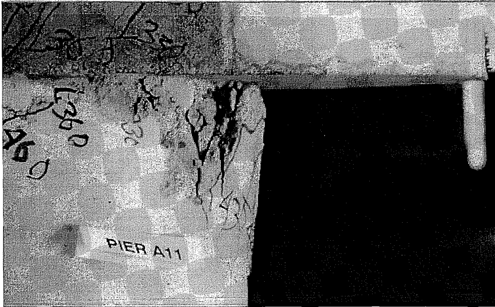
Figure 3.6 Crushing of Pier A1-1 After Failure
