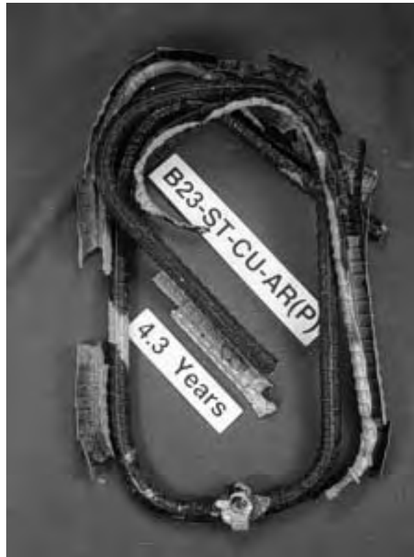
Figure 1.14 Coating extensively debonded on stirrups from beam specimens. 34
