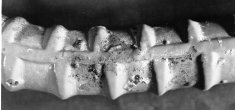
Figure 4.2 Corrosion at blisters on coated bars
