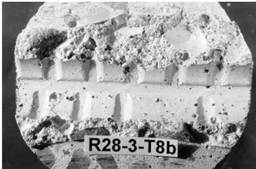
Figure 4. 21 Typical distribution of voids under rebar
