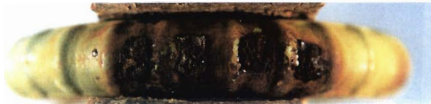
(b) Corrosion in exposed areas
