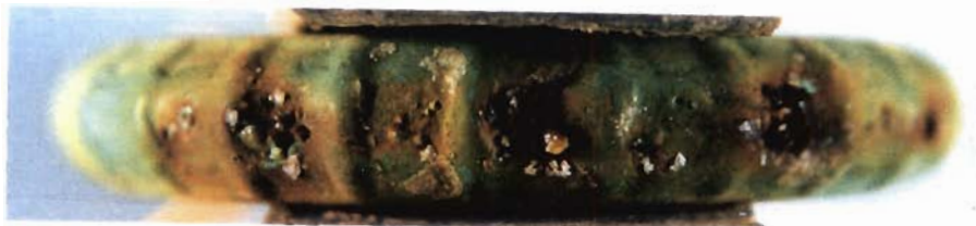
(a) Corrosion in patched areas
