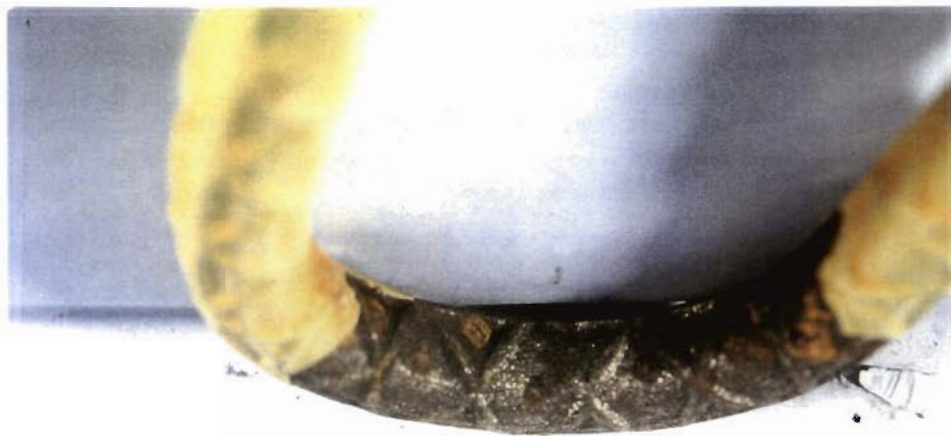
(b) The inside of bend of the bar shown in Figure 3.16(b)
