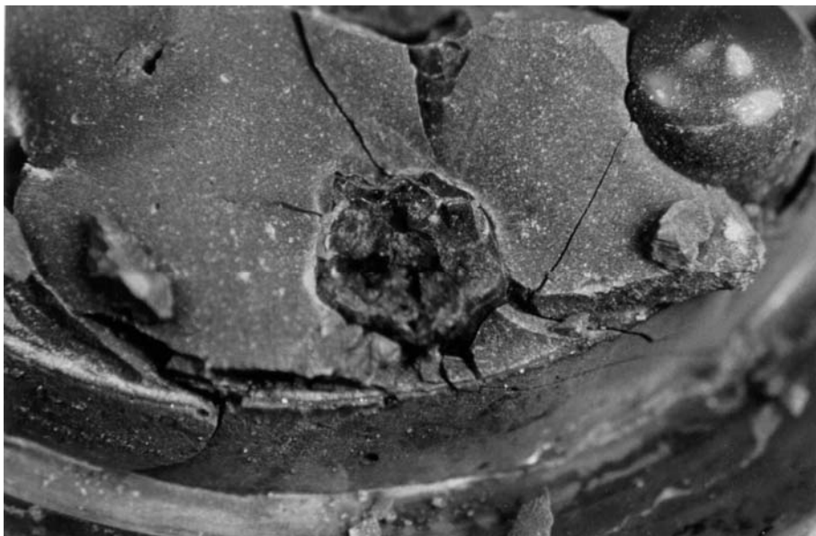
Figure 8- 34 Corroded end of strand repaired with epoxy compound
