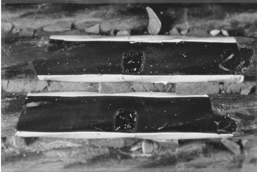
Figure 8- 39 Repaired damage location after completion of corrosion test
