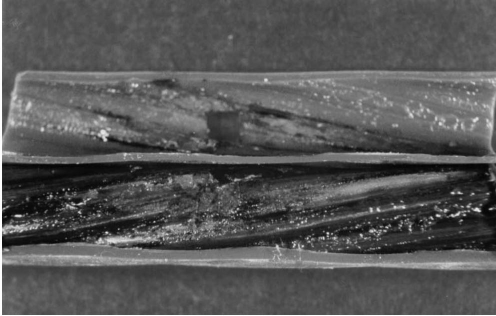
Figure 8- 37 Corrosion under sheathing
