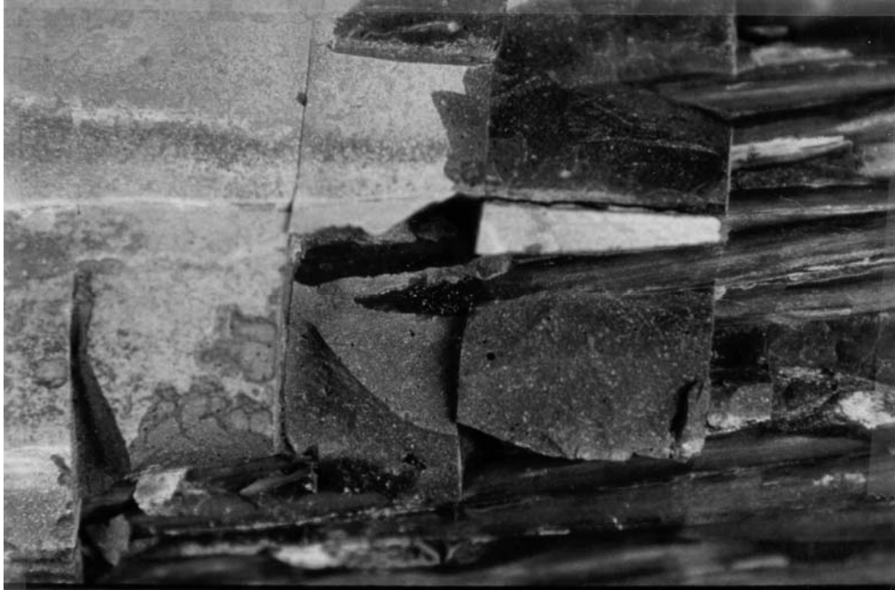
Figure 8- 19 Typical corrosion at base of a grout crack
