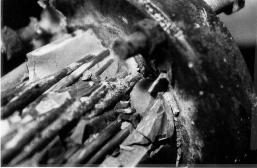
Figure 8- 26 Corrosion of strand adjacent to deviator ring
