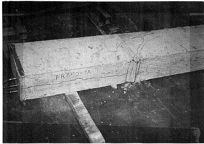
Figure 4.18 Photograph of Cracking at Failure Beam FR350-1 Test A: Bond Failure
