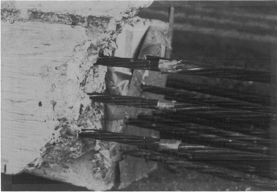
Figure 6.4 Portion of the strands in the transfer zone after removal of concrete.
