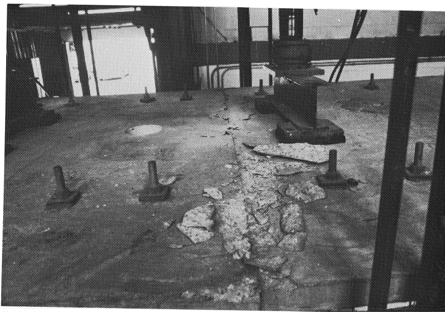
Figure 3.70 Crushing of top flange in epoxy joints span.
