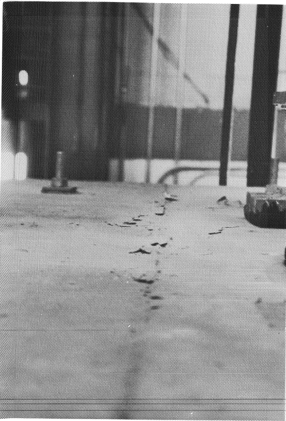
Figure 3.120 Crushed critical joint top flange.
