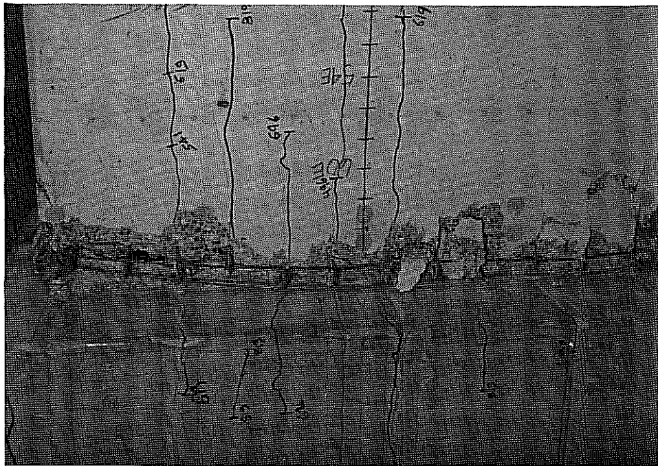
Figure 3.28: Specimen 4M18 Compression Flange Close-Up
