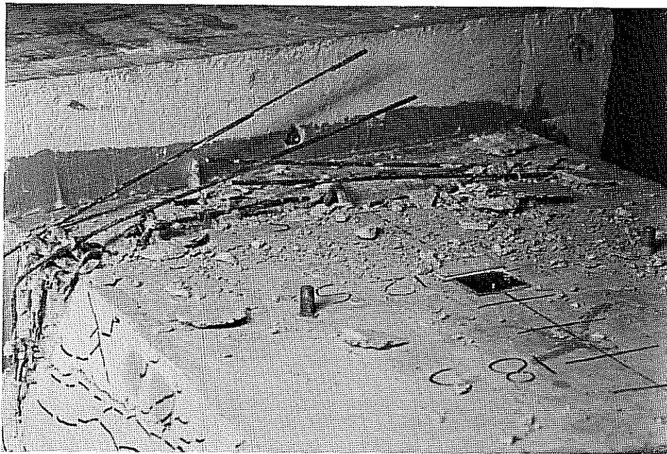
Figure 3.103: Specimen 12S29 Side Face Close-Up
