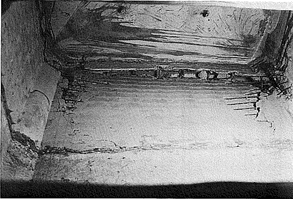
Figure 3.100: Specimen 12S29 Interior View of Failure Region
