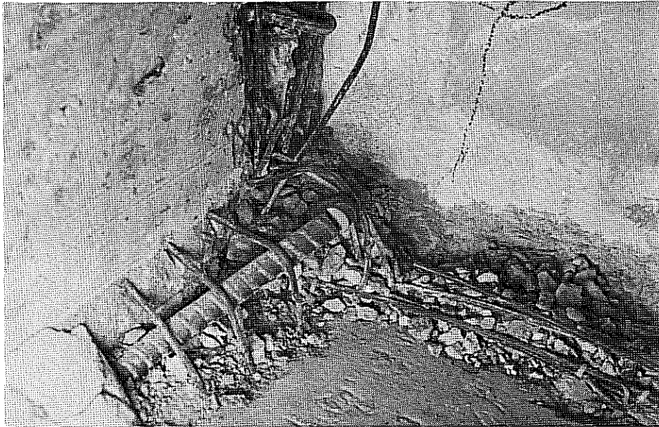
Figure 3.52: Specimen 7S22 Interior View of Post-Tensioning Bar
