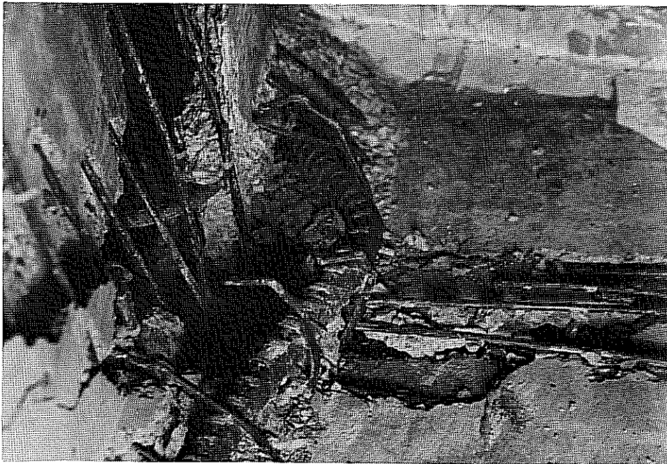
Figure 3.101: Specimen 12S29 Interior View of Post-Tensioning Bar
