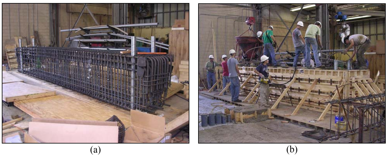
Figure 3.22: Fabrication of a 36''x48'' beam: (a) tied reinforcement cage (b) placement of concrete into wooden formwork
