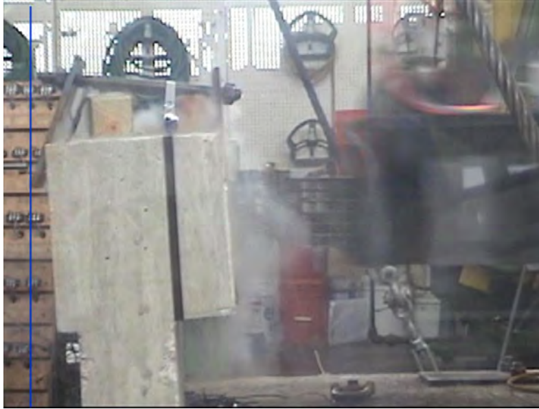
Figure 8.1: Still image from impact pendulum test on stand-alone, cast-in-place T203 bridge barrier and deck specimen
