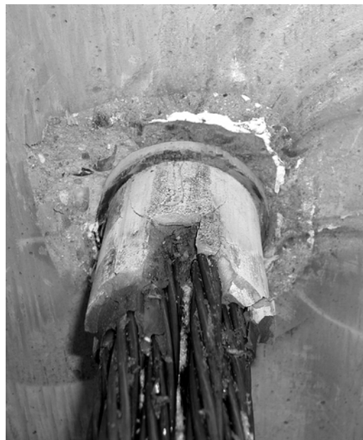
Figure 5-16 Live End of Specimen 1-SP-7.5°-2 after Testing
