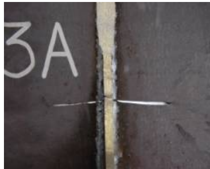
Figure 4-15: Crack at Upper Radial Web Taper
