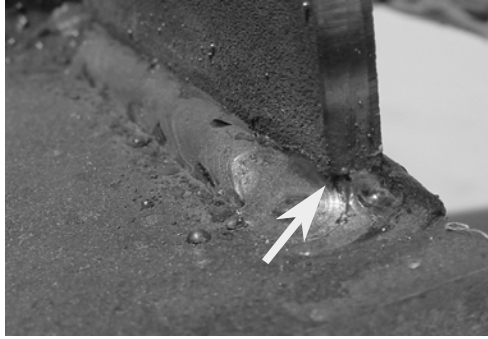
Figure 2-21: Specimen A Stiffener Corner Undercut
