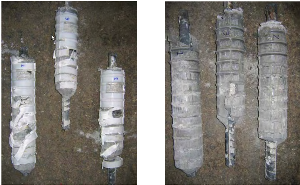
Figure 6.31 Connectors from Test 32 after Pullout (Polypropylene Duct)
