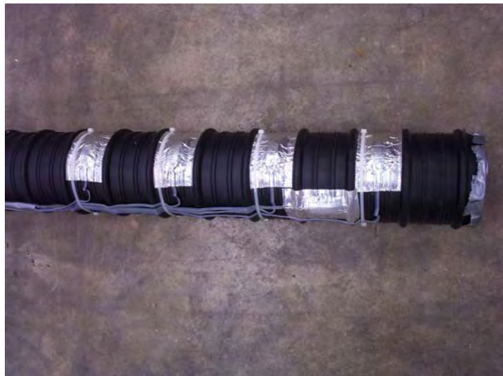
Figure 5.6 Completed Gage Installations on HD Polyethylene Duct
