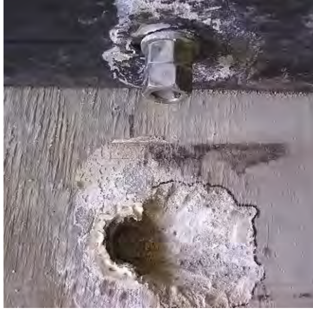
Figure 4.7: Failed Specimen DBLNB-56HF
