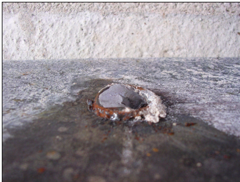
Figure 3.22: Typical failure of welded stud above the weld pool
