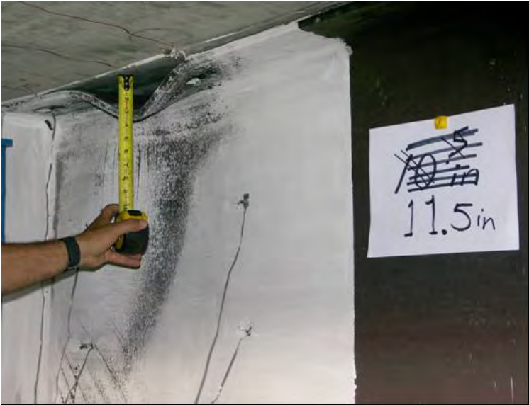
Figure 5.22: Typical beam local flange and web buckling at large displacements
