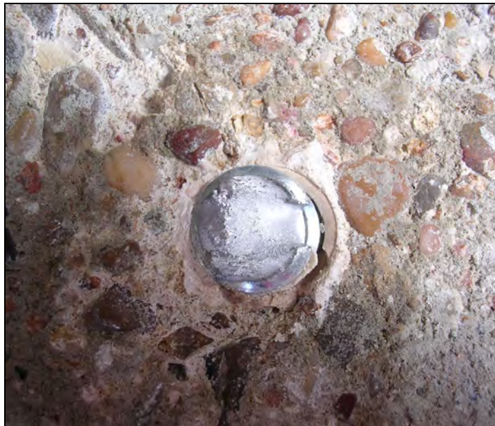
Figure 3.24: HAS-E adhesive anchor failure at the shear plane
