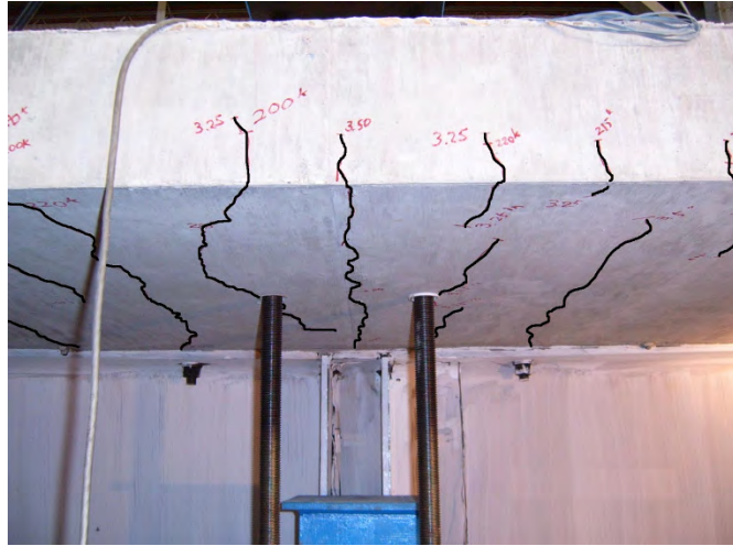
Figure 5.17: Specimen DBLNB-30BS—Cracks on the bottom of the concrete slab (3.25-in deflection)
