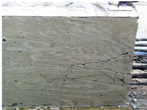
Figure 5-8: Cracking at release end due to bursting stresses (R2-75-2)
