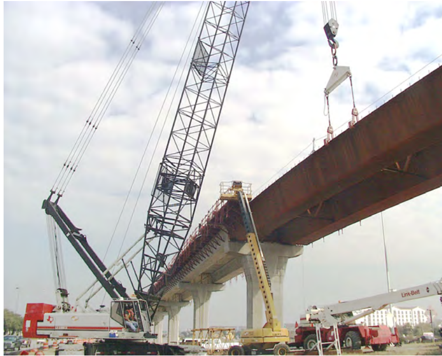
Figure 3.4 Loading Crane & Top-Flange Attachment
