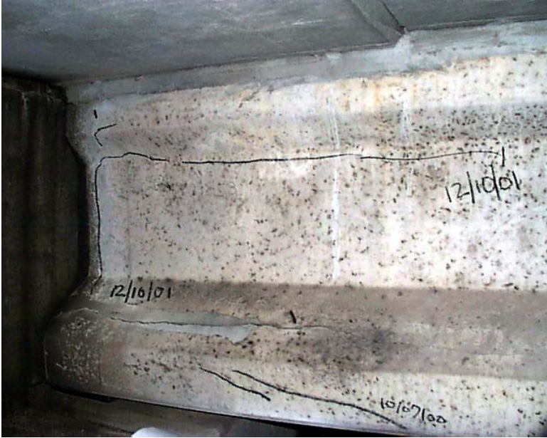
Figure 7.7: New cracks on south face of SW Girder 3 at west abutment, I-10 (12/10/01)
