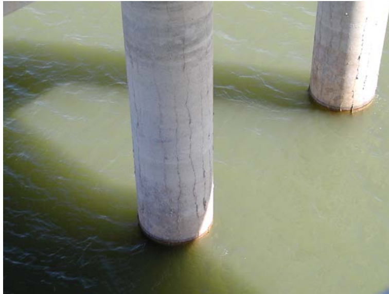
Figure 7.44: Example of column cracking near waterline of Bent 5 (4/24/01)
