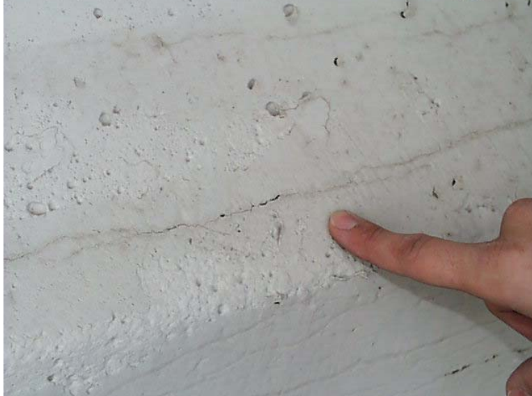
Figure 7.14: Apparent cracking through sealant, US-90 (12/11/01)
