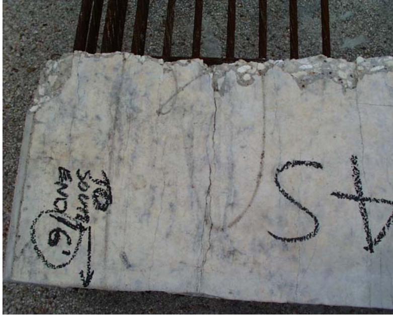
Figure 3.17: Cracking on bottom face of Slice BG4S1
