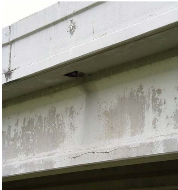
Figure 7.10: Typical crack under drain at US-90 structure (10/6/00)
