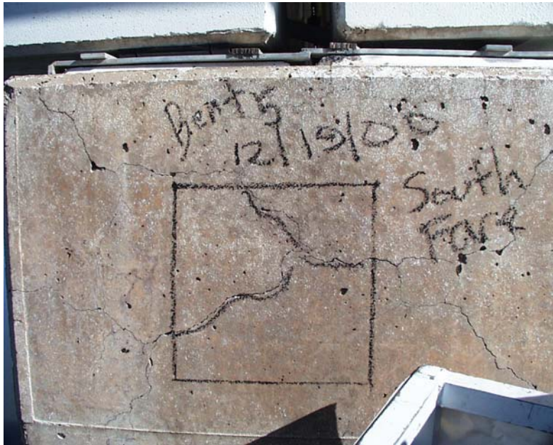
Figure 7.42: 12 in. (0.31 m) square on south end of bent cap, Bent 5 (12/19/00)
