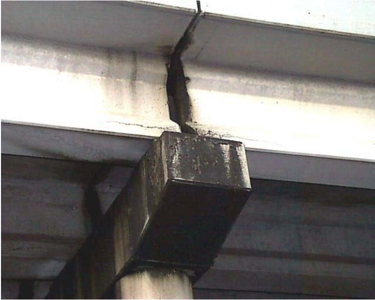
Figure 7.8: Cracks at first bent east of west abutment, I-10 (12/10/01)
