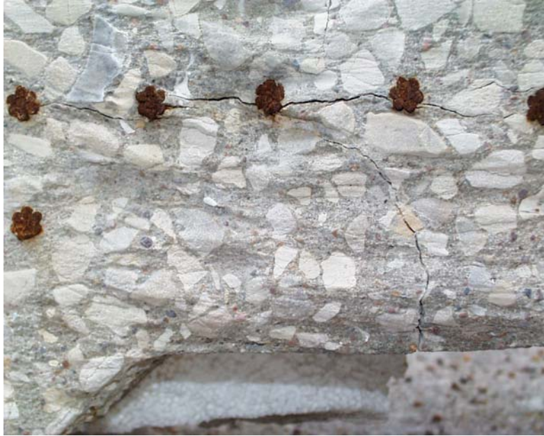
Figure 3.19: Damage to cross section of Slice BG4S1 (back face)
