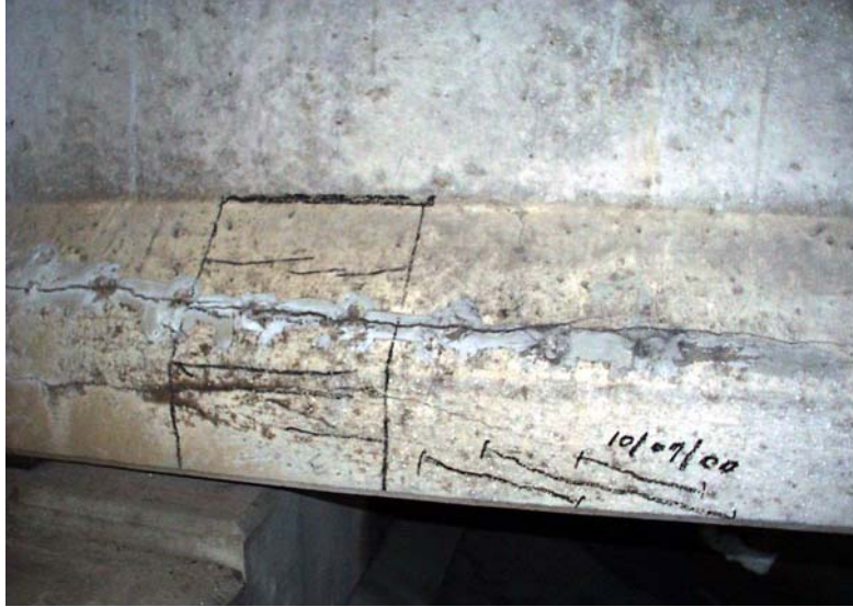
Figure 7.4: Representative areas on I-10 SW Girder 2, south face (10/7/00)
