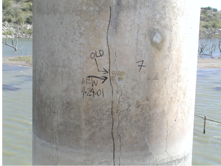
Figure 9.11: Typical vertical cracking on south lower column of Bent 5 (10/15/01)
