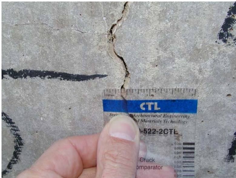
Figure 7.50: Close-up of vertical cracking at Point 10 near waterline, Bent 11 (10/15/01)
