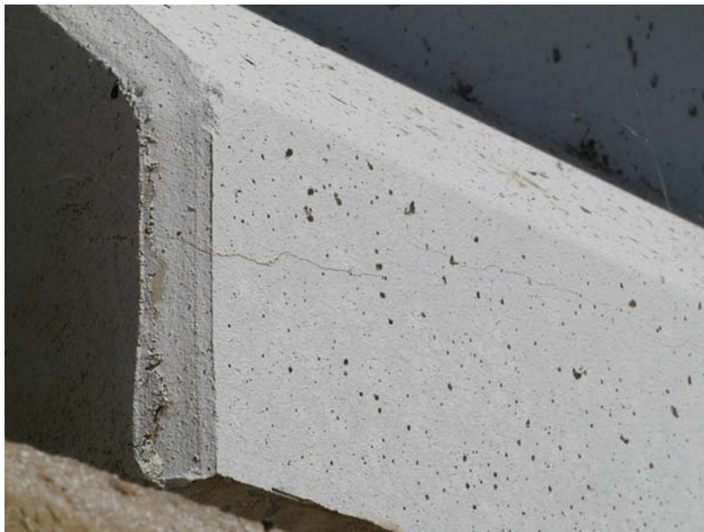
Figure 7.48: Close-up of new cracks on south girder at Bent 9 (10/15/01)
