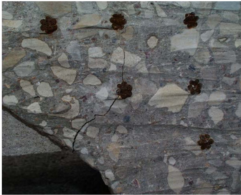
Figure 4.7: Crack in back of Slice BG4S1 at Strand 17R (Center)
