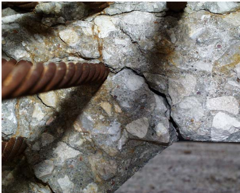
Figure 3.22: Front view of right inside corner of Slice BG4S2
