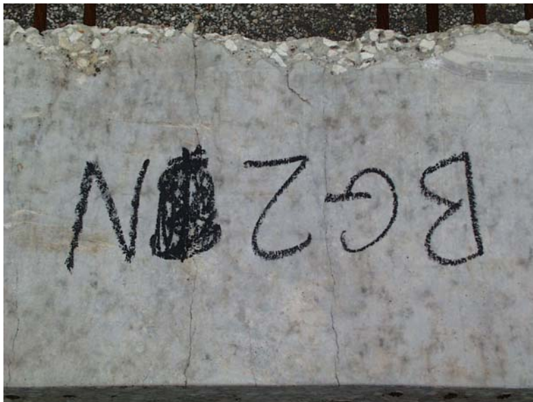
Figure 3.16: Cracking on middle of bottom face of Slice BG2N
