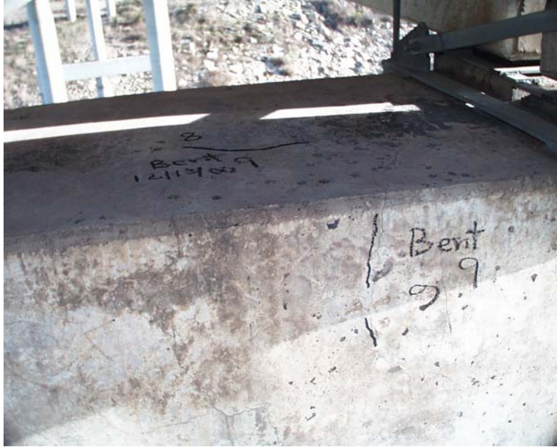
Figure 7.41: Cracking on bent cap, Bent 9 (12/18/00)
