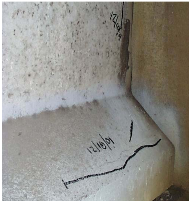
Figure 7.22: New cracks on north surface of NW Girder 3, Robinson Road, at west abutment (12/10/01)
