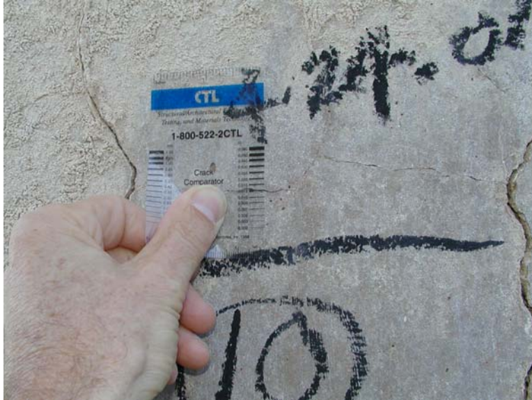
Figure 7.51: Close-up of horizontal crack at Point 10 near waterline, Bent 11 (10/15/01)
