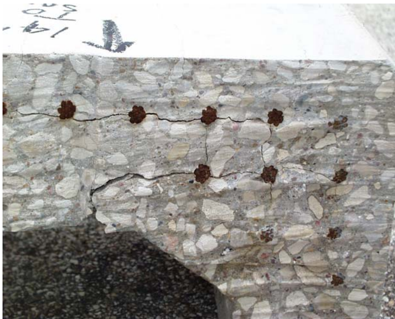
Figure 3.20: Cracking in back face of Slice BG4S2
