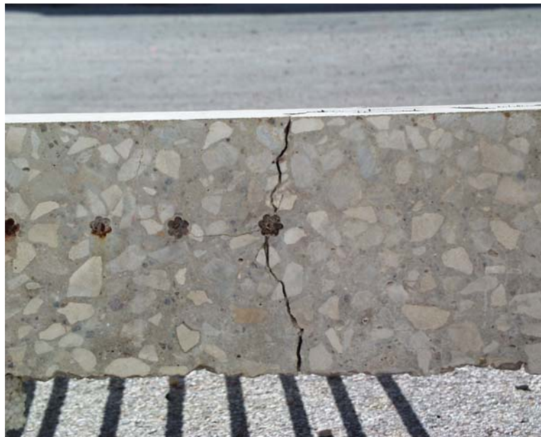
Figure 3.11: Crack through Strand 9L in back face of Slice BG1S
