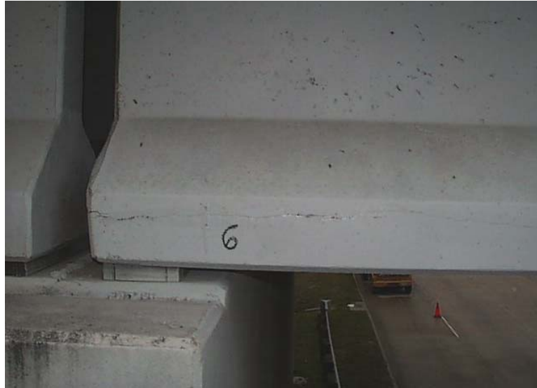
Figure 7.30: Cracking near Point 6, Beltway 8 structure (12/11/01)
