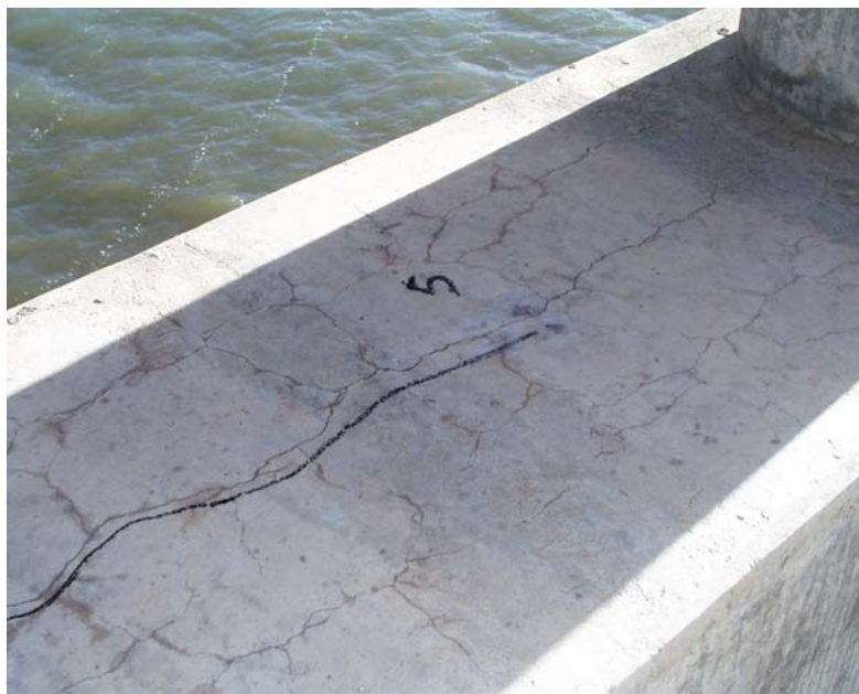
Figure 7.40: Map cracking on tie beam, Bent 5 (12/18/00)
