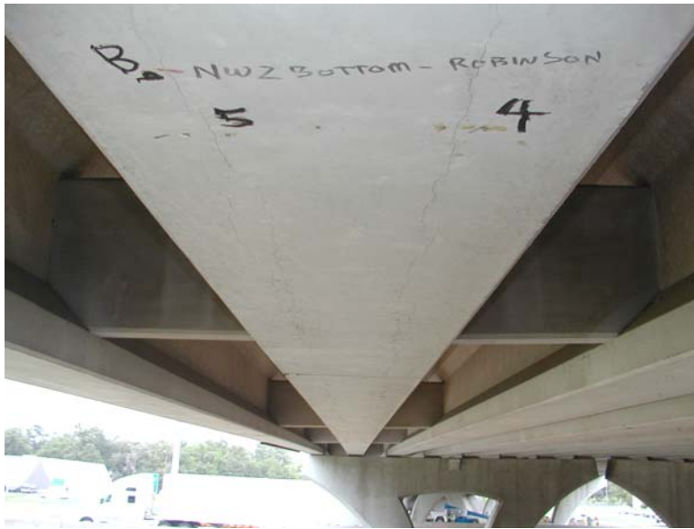
Figure 7.18: Extension of cracking on underside of NW Girder 2, Robinson Road (6/21/01)
