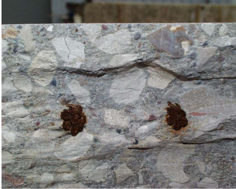
Figure 4.11: Back view of Strand BG4S1_4R (right) and Strand BG4S1_5R (left)
