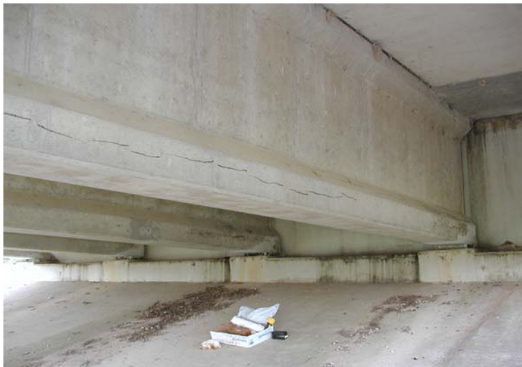
Figure 7.11: Extension of existing cracking on north surface (Face 5) of NW Girder 2, US-90 (6/22/01)
