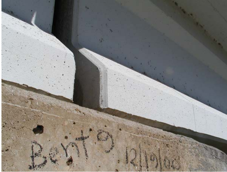
Figure 7.47: New cracks on exterior faces of south girders at Bent 9 (10/15/01)
