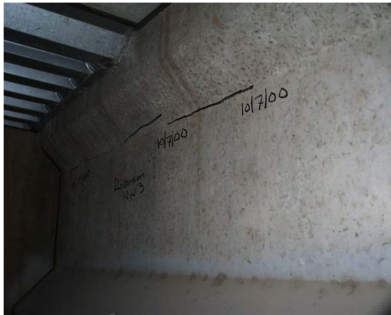
Figure 7.16: Extension of new cracking on south face of NW Girder 3, Robinson Road (10/7/00)
