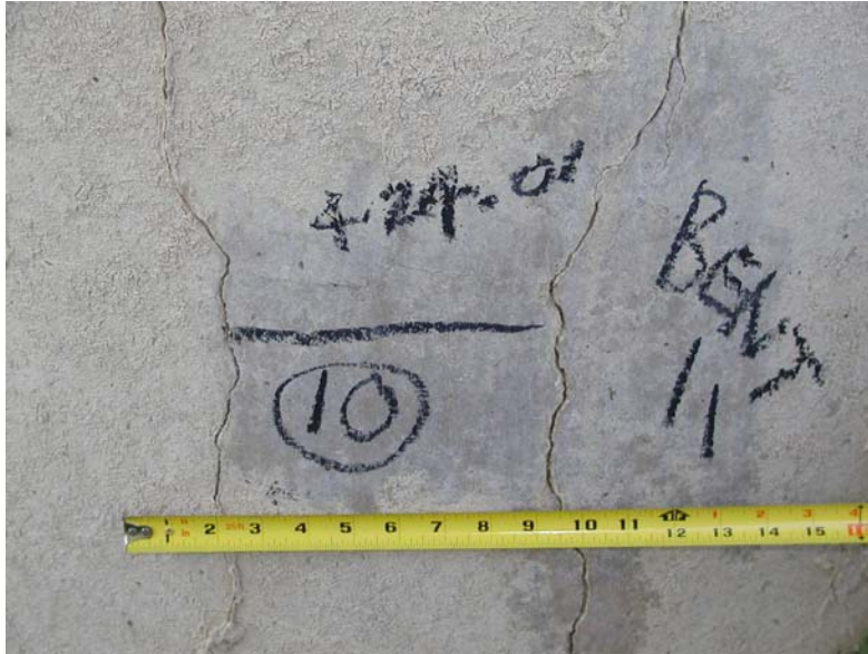
Figure 7.49: Column cracking at Point 10 near waterline, Bent 11 (10/15/01)
