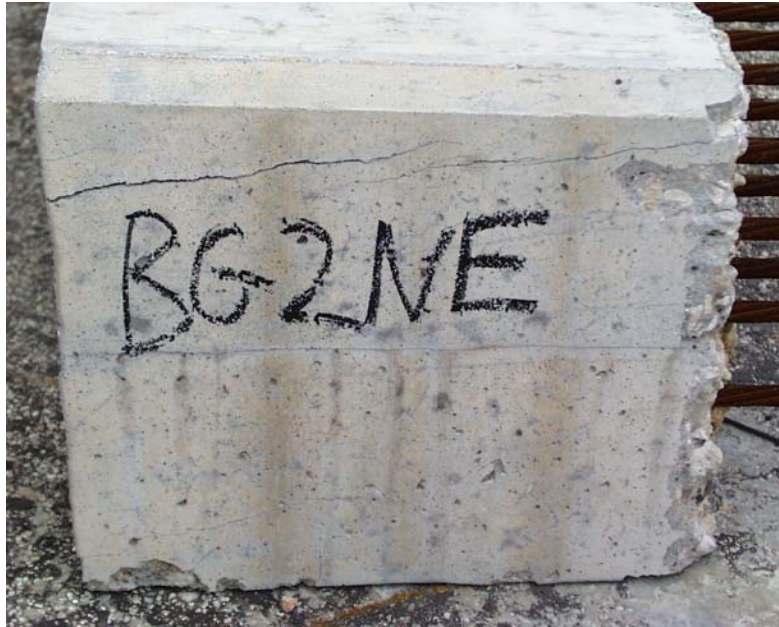
Figure 3.14: Cracking on right face of Slice BG2N
