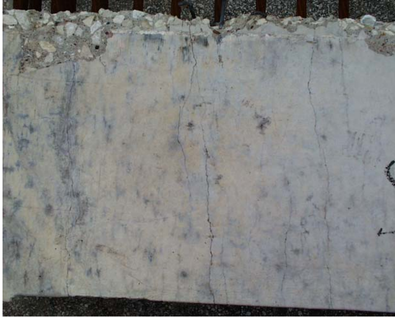
Figure 3.21: Cracking on bottom face of Slice BG4S2
