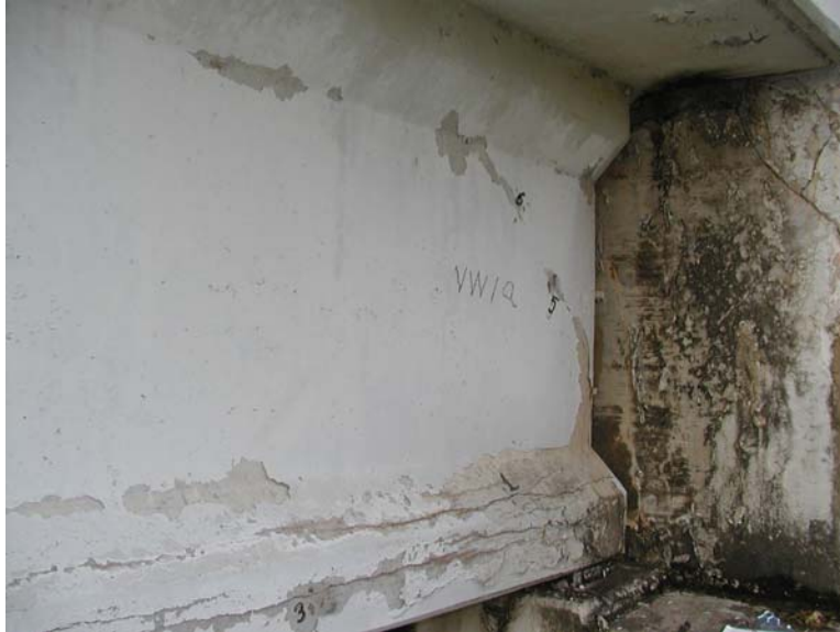
Figure 7.12: Cracks at end of NW Girder 1, US-90 (6/22/01)
