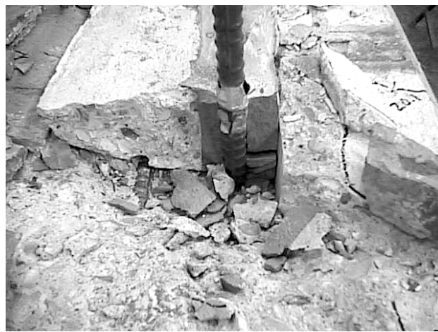
b. Spalling above DL04 Confinement
