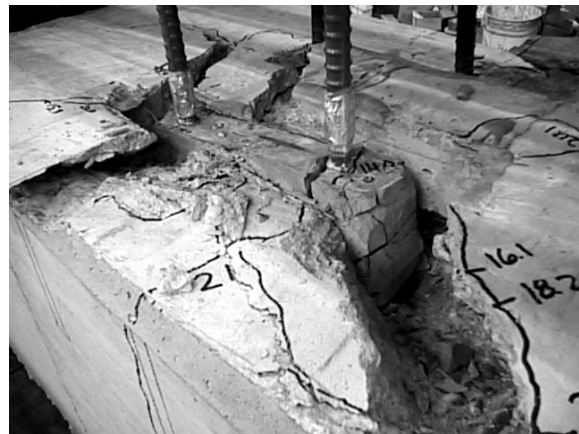
b. Exposed Surface Spalling
