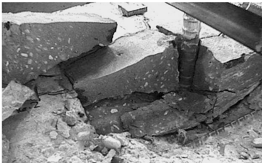
Figure 3.25 Dye Injected into Air Voids
