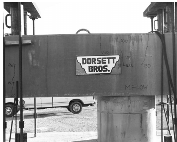
Figure 5.44 Flexural Cracks for CB1
