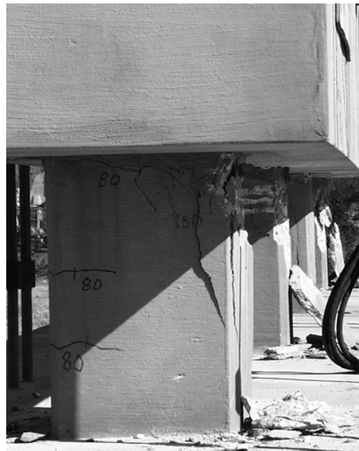
Figure 5.41 Crushing and Spalling at Pile Tops in PB3—Side View
