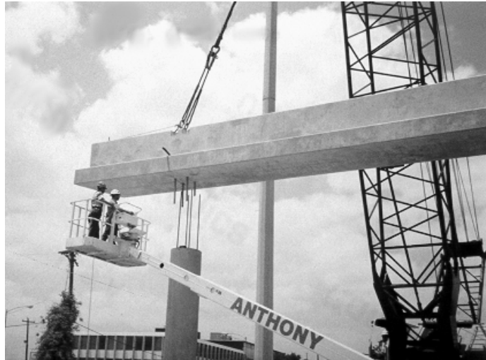
Figure 1.6 Workers Prepared to Thread Dowel Bars through Precast Bent Cap with Aid of Extended Pipes
