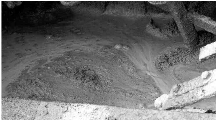
a. Bubbling of Grout
