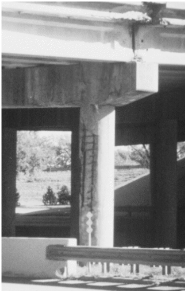
(a) Deicing Chemical Exposure “Attack from Above”
