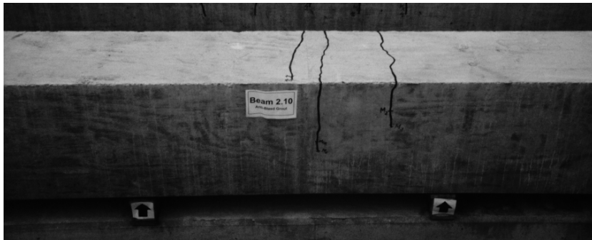
Figure A.44 - Crack Pattern for Specimen 2.10
