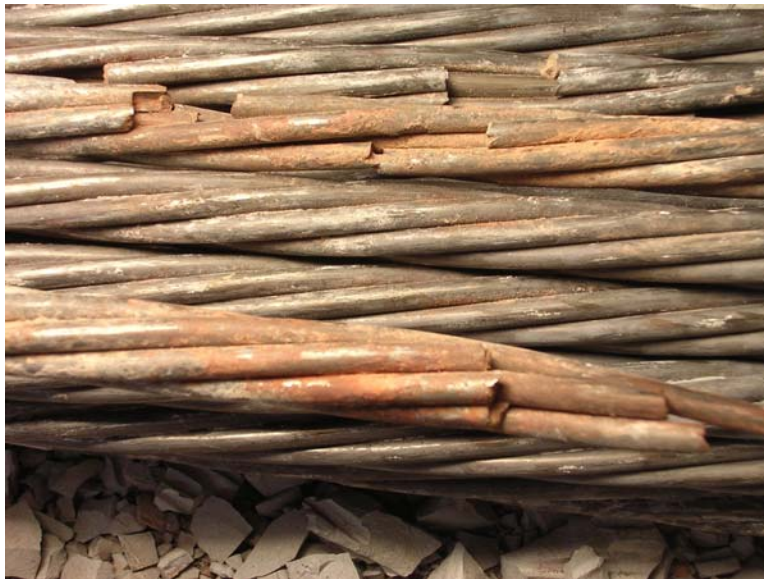
Figure D.109 Corrosion on Surface of Strand near Midspan – Specimen 9
