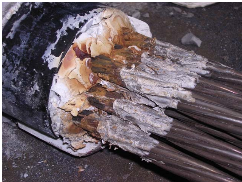
Figure D.93 Corrosion Product Observed at Interface between Caulk and Grout in Specimen 8
