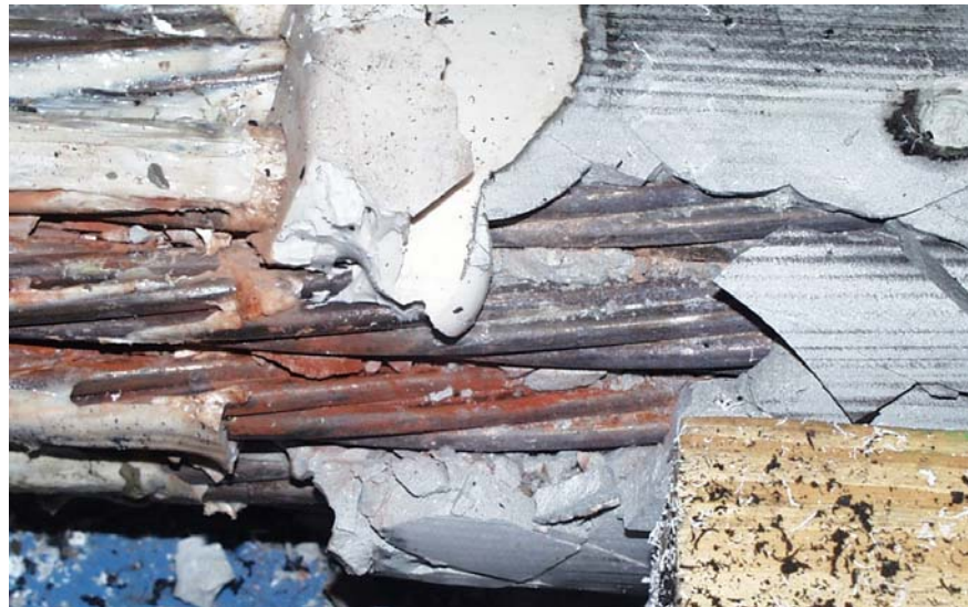
Figure D.51 Corrosion Product Observed at Interface between Caulk and Grout in Specimen 5
