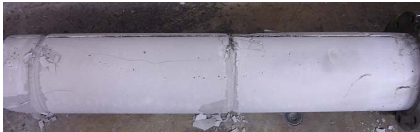
Figure D.134 Condition of Grout at Tower End – Specimen 11
