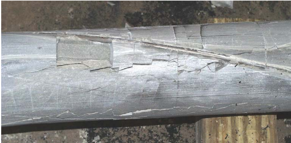
Figure D.59 Grout near Midspan of Specimen 6
