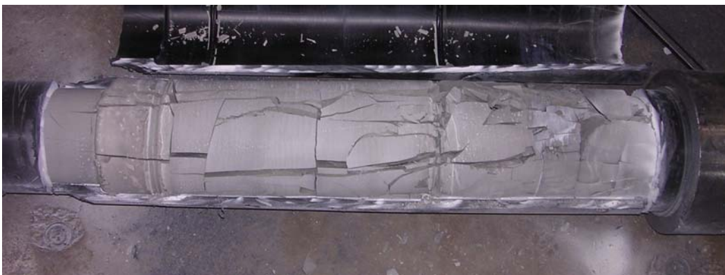
Figure 3.10 Condition of Grout at Deck End Immediately after Removing PE Pipe – Specimen 10
