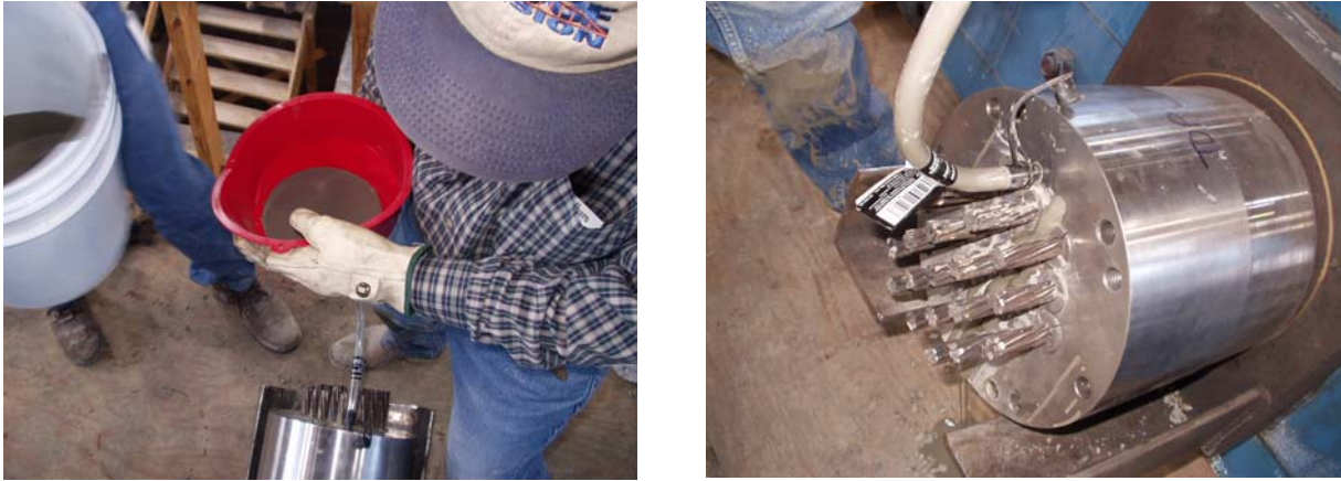
Figure B.39 Procedure Used to Fill the Intentional Grout Void at the Tower End of Specimen 9
