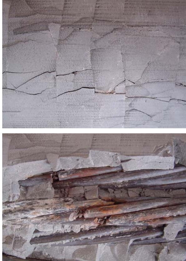
Figure D.8 Longitudinal Cracks in Grout, Corrosion of Strand, and Wire Breaks near Midspan of Specimen 1
