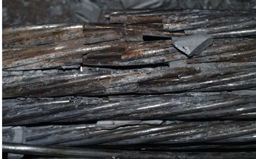
Figure 3.9 Corroded Fretting Product on Surface of Strand at Midspan – Specimen 12
