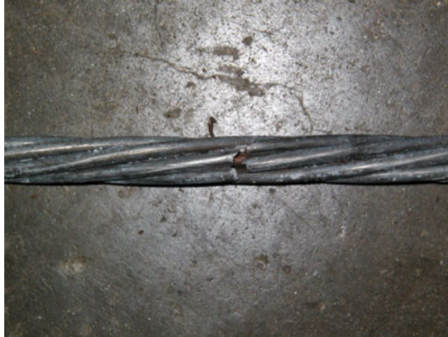
Figure E.8 Wire Breaks near Midspan – Specimen 1
