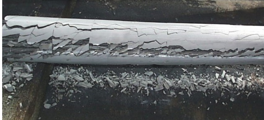
Figure D.121 Condition of Grout at Midspan Immediately after Removing PE Pipe – Specimen 10
