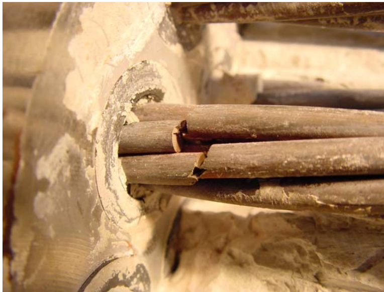
Figure D.14 Wire Breaks in Strand 2 near Tower End of Specimen 1
