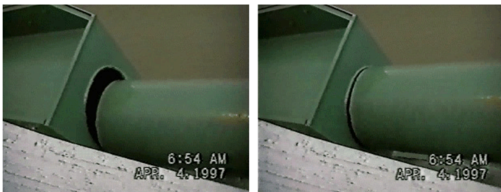
Figure 1.5 Broken Guide Pipe – Fred Hartman Bridge
