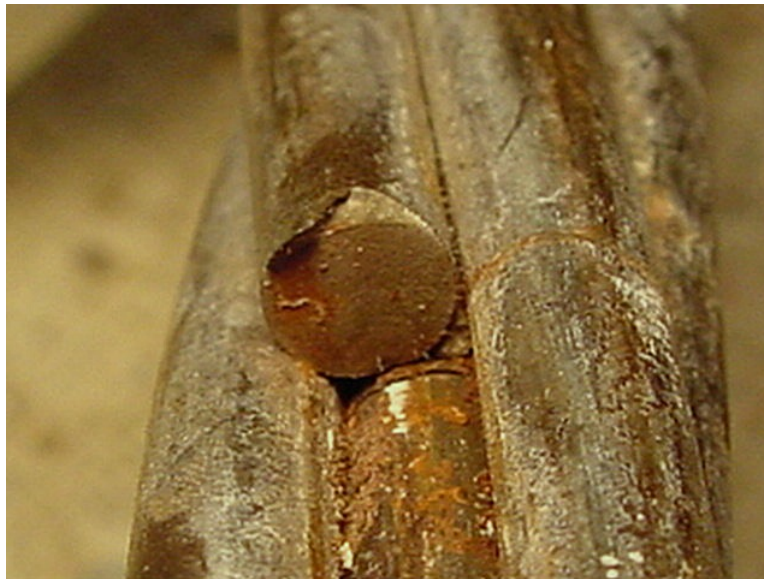
Figure D.30 Detail of Fractured Wires shown in Figure D.29
