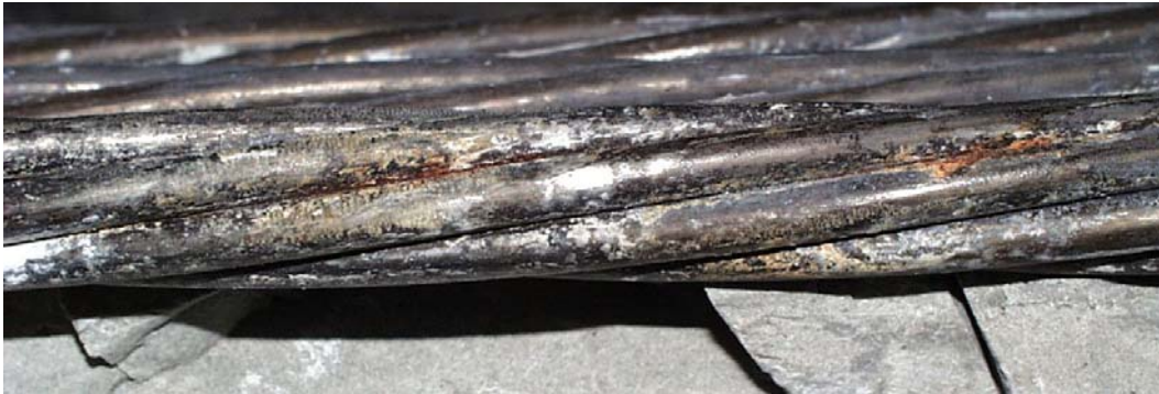
Figure D.61 Corrosion on Strand 19 near Tower Anchor Head – Specimen 6
