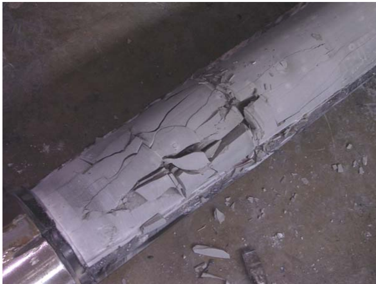
Figure D.120 Condition of Grout at Tower End Immediately after Removing PE Pipe – Specimen 10
