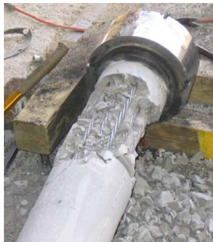
Figure D.74 Condition of Grout near Deck Anchor Head Several Minutes after Removing Polyethylene Pipe – Specimen 7
