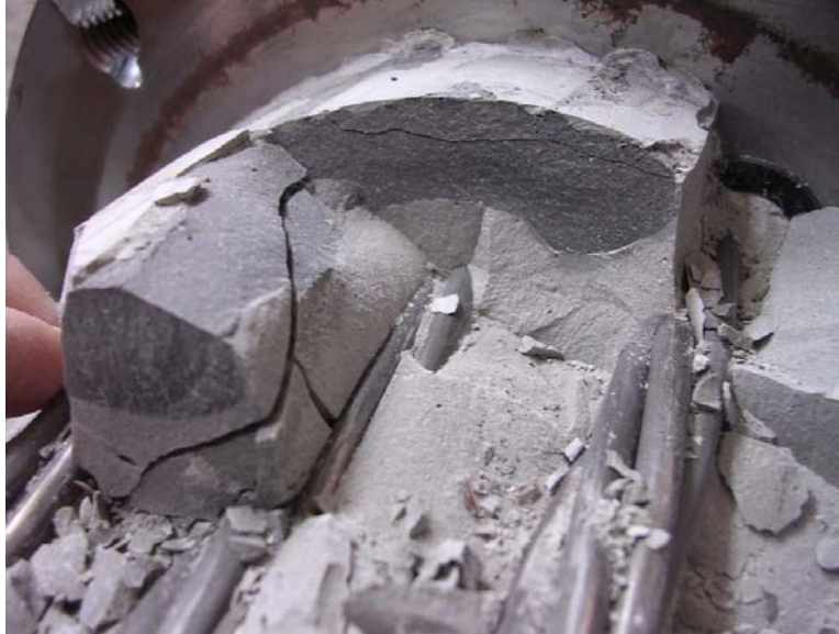
Figure D.106 Interface between Grout Used to Construct Specimen 9 and Grout Used to Repair Intentional Void at Tower End
