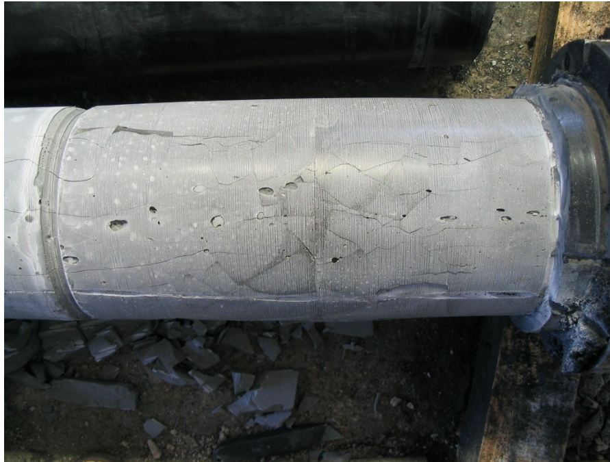
Figure D.72 Condition of Grout at Tower End - Specimen 7
