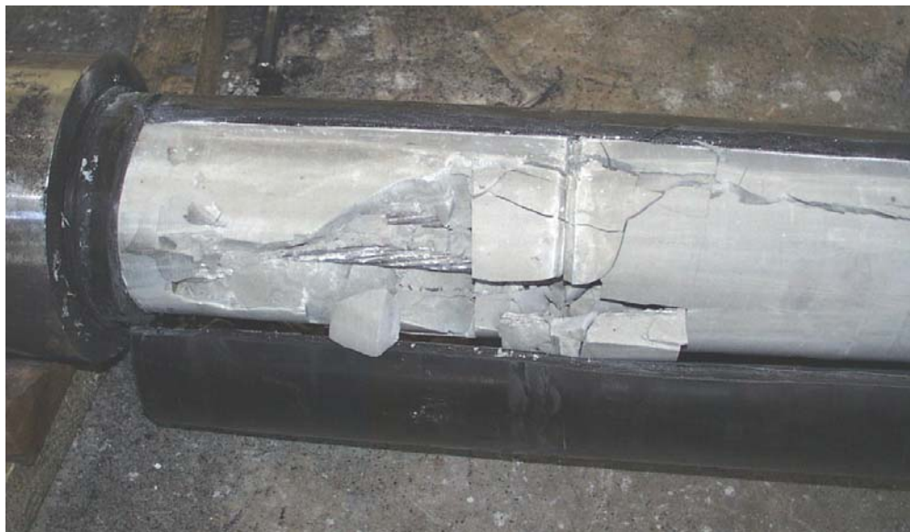
Figure D.58 Grout Cracking near Tower End – Specimen 6
