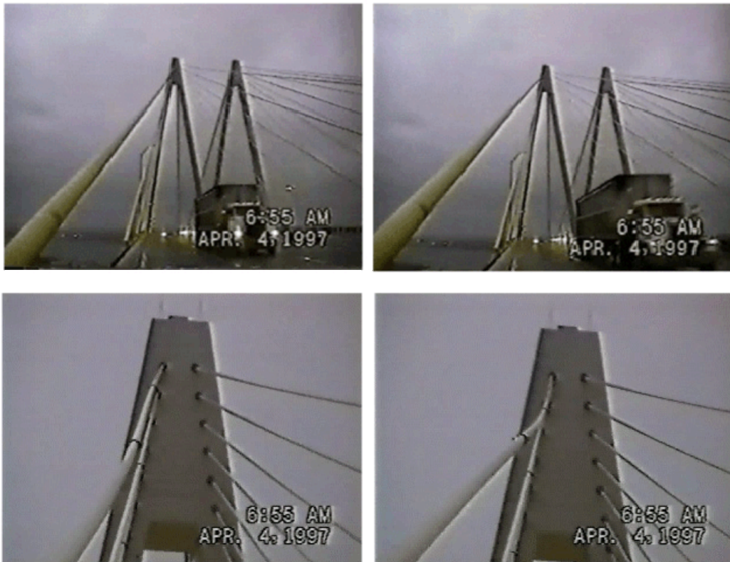
Figure 1.4 Stay Cable Vibrations – Fred Hartman Bridge
