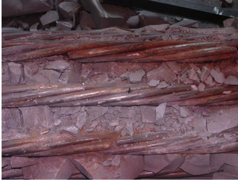
Figure D.123 Corroded Fretting Product near Tower End – Specimen 10
