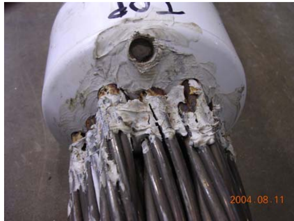
Figure D.137 Corrosion at Interface between Grout and Caulk near Midspan – Specimen 11
