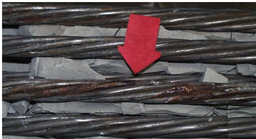
Figure D.151 Black Corrosion on Surface of Strand near Tower End – Specimen 12
