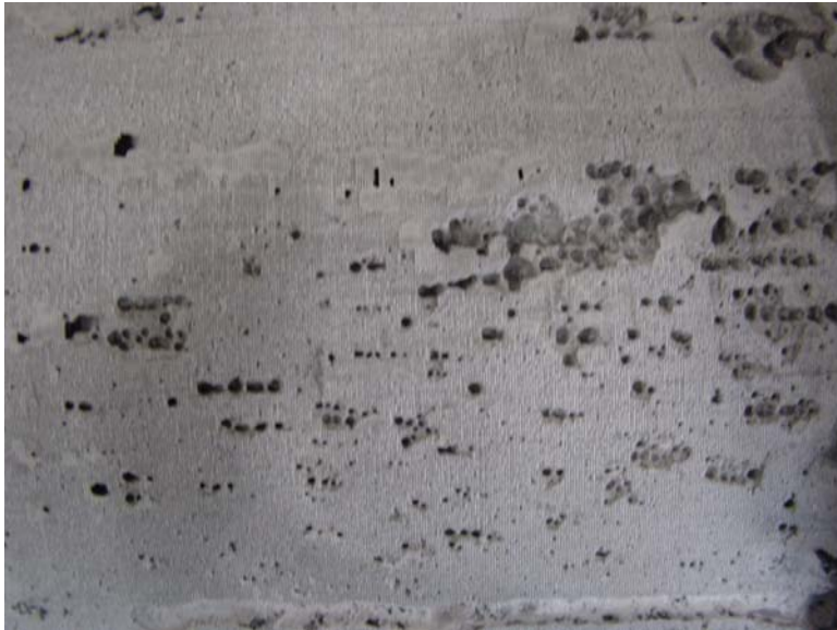
Figure D.20 Air Voids in Grout near the Deck End – Specimen 2
