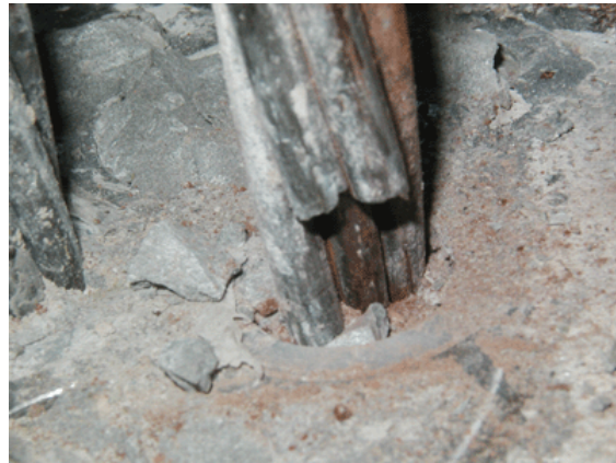
(b) Wire Breaks in Bottom Strand outside Anchor Head
