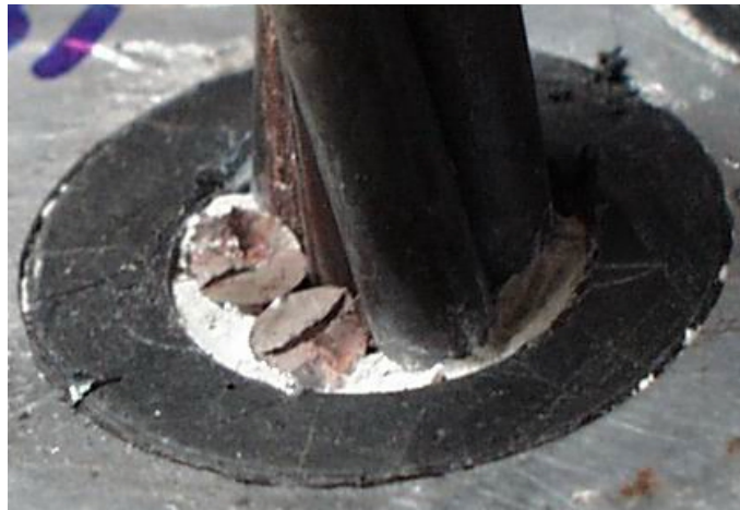
Figure D.66 Wire Breaks in Strand 17 at the Inside Face of the Tower Anchor Hear – Specimen 6
