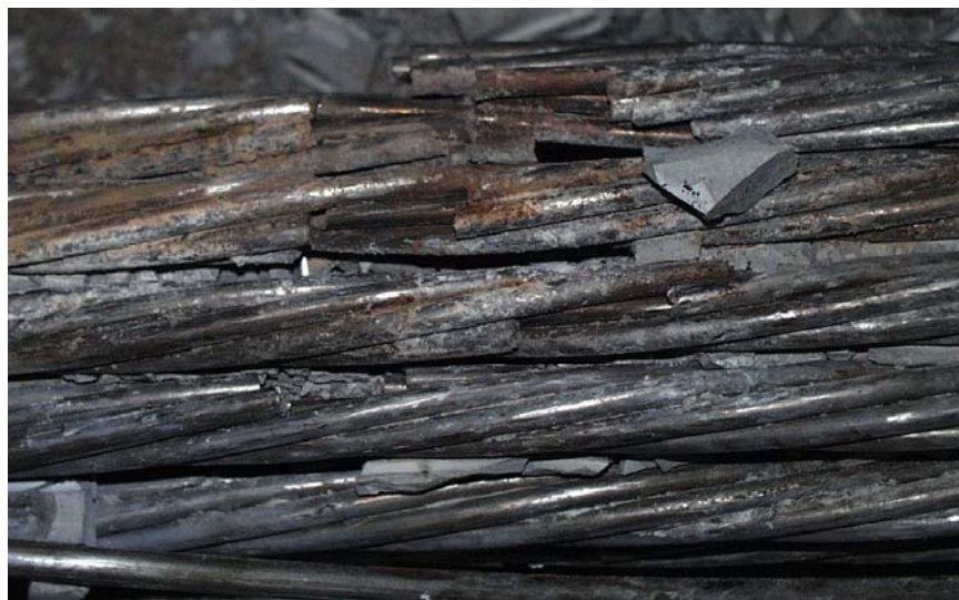
Figure D.148 Corroded Fretting Product on Surface of Strand at Midspan – Specimen 12
