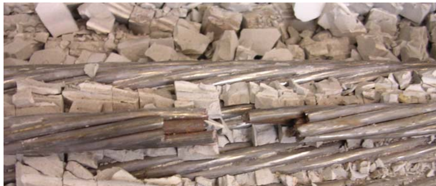
Figure D.138 Corroded Fretting Product on Surface of Strand 18 at Midspan – Specimen 11
