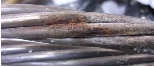
Figure D.108 Corrosion on Surface of Strand near Tower End – Specimen 9
