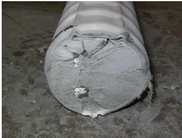
Figure E.9 Typical Vertical Crack in Grout – Specimen 1
