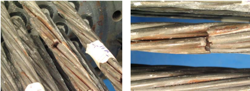
Figure D.76 Corrosion Observed near Tower Anchorage on Strand 18 – Specimen 7
