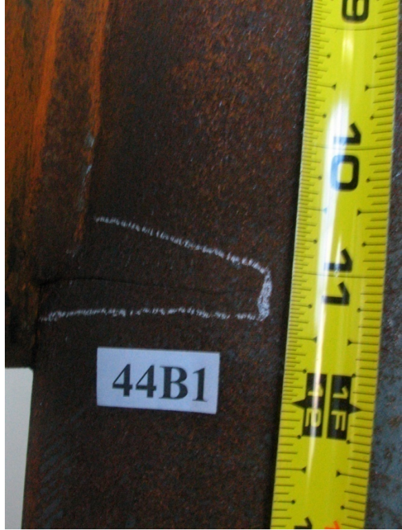
Figure 42. 44B Angle Failure Backside Close-Up
