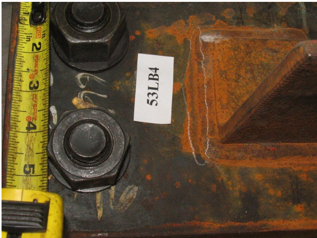
Figure 53. 53LB Angle Failure Close-Up
