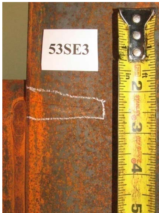
Figure 46. 53SE Angle Failure Close-Up
