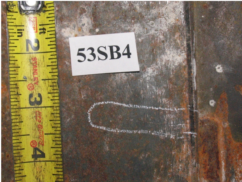
Figure 48. 53SB Failure Close-Up
