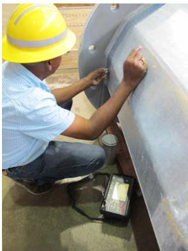
Ultrasonic test conducted to characterize the weld cracks in the shaft-to-base plate connection
