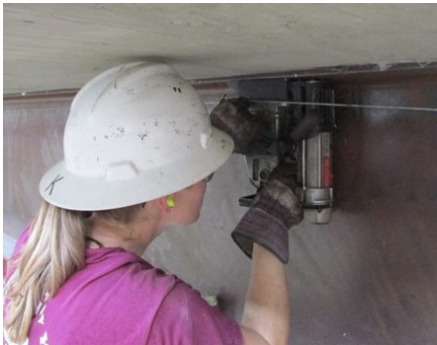
Installing the adhesive anchors: Drilling holes (left) and inserting the threaded rod (right)
