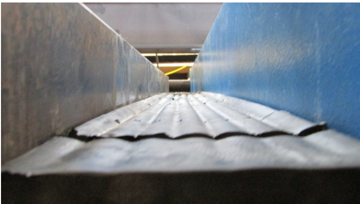
This is how one bearing "reacted" to a two-million pound compressive force
