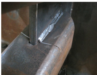
Z frame HSS fatigue cracks show stress concentration at connection
