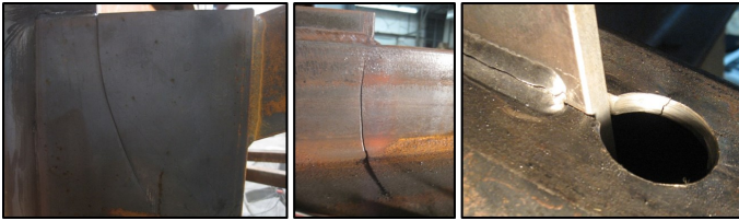
Examples of fatigue cracks in X frame (far left), K frame (center), and Z frame with HSS tubes (right)
