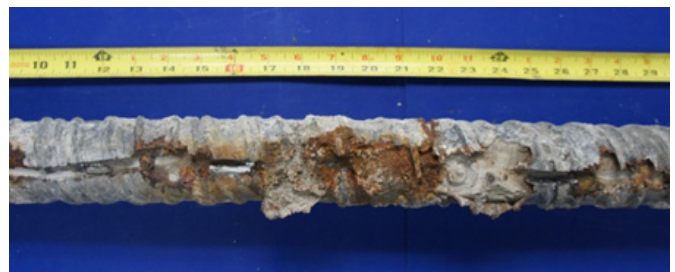
Galvanized Duct + Chlorides = Corrosion
