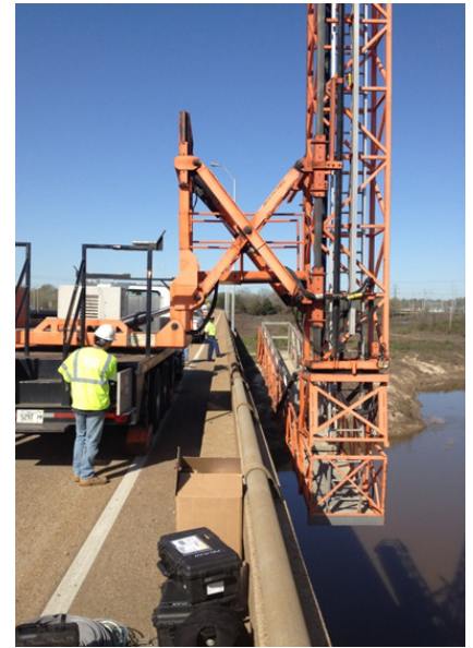
“MOOG” - def. moveable platform used to access the bridge girders from the top of the bridge deck
