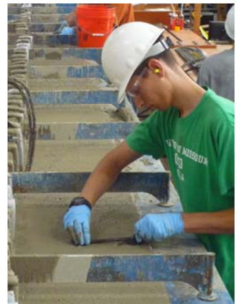
DPL setting the hangers into the concrete beam for the overhang brackets
