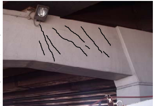
Use of the STM provisions would have predicted such diagonal cracking
