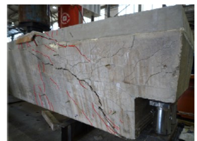
An example of Atrociously Bad Cracking and Delayed Ettringite Formation (ABC/DEF)
