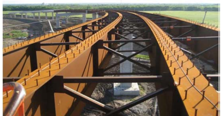
Figure 1: Cross-frames in Horizontally Curved I-girder Bridge (Direct connector between SH 71 and SH 130 in Austin Texas)
