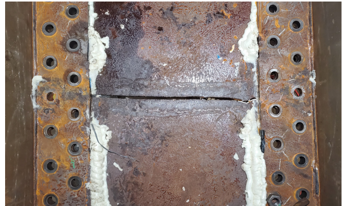
Fractured bottom flange plate of specimen with cross-boundary separation (after ultimate strength test)
