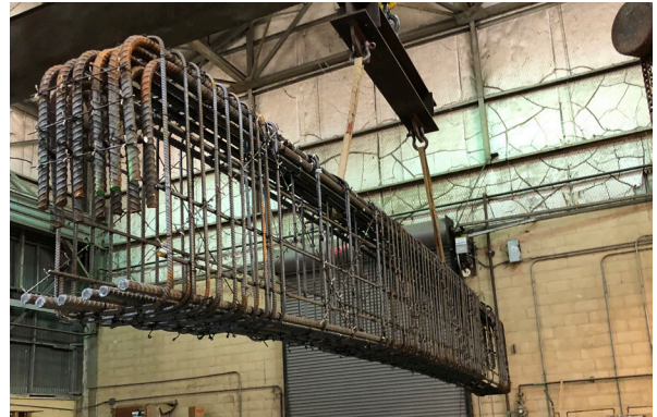
Rebar cage for first specimen being lifted into the formwork for cast
