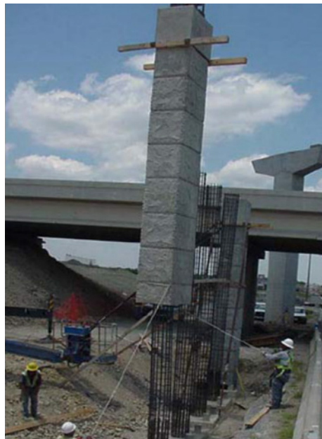
Precast shell system being installed in Waco, TX, like the system being investigated.
